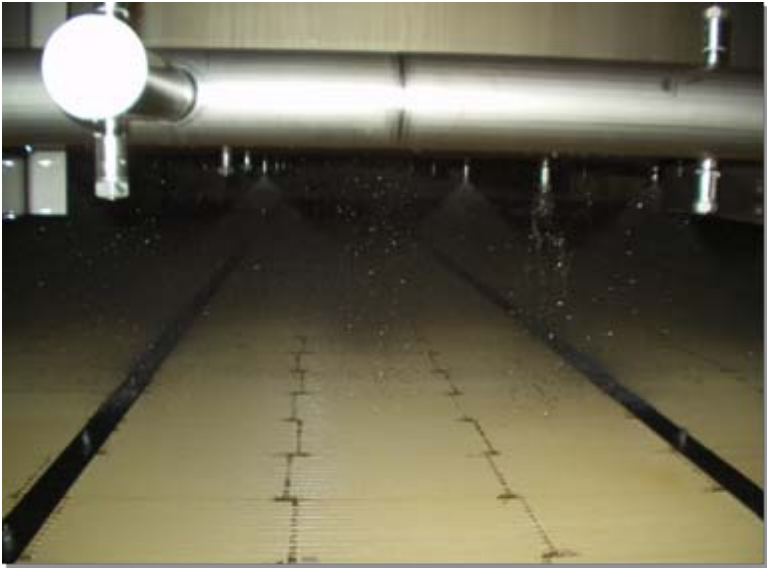
Mist Eliminator Wash System
