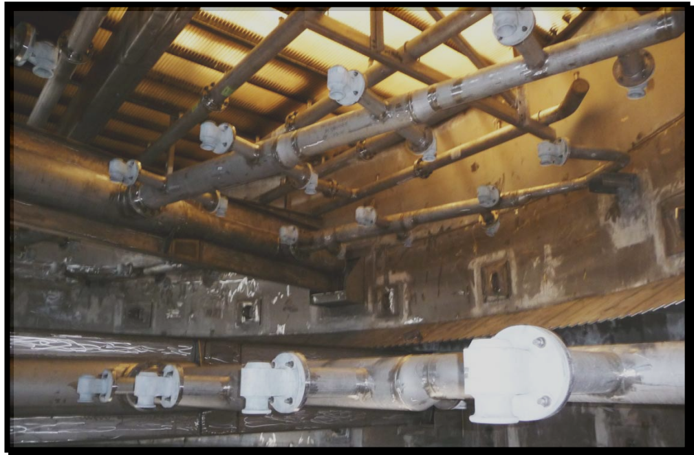
Absorber Spray Levels
