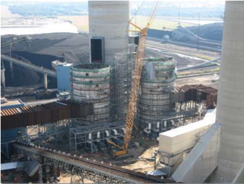
Fayette Power Project, Units 1, 2 and 3 Texas
